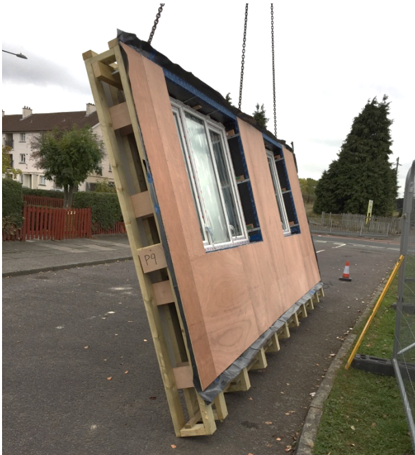
Figure 5: External insulation panel built from timber frame, before installation and insulation injection.
