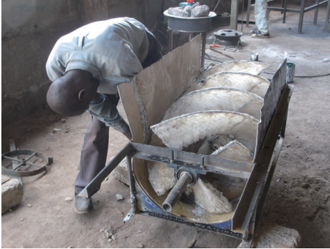
Fig. 4. Blades and housing of the screw turbine
