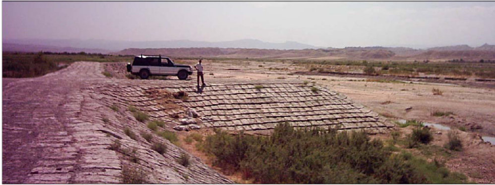
Figure 1-4. An spur dike with trapezoidal shape cross section at Sarakhs river, Iran (Yasi 2009)
