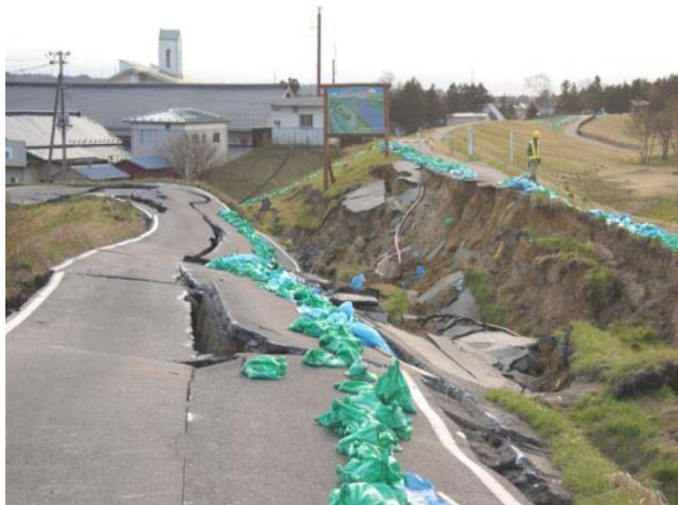
Figure 1.3. Major slumping of landside slope of Naruse River dike at river kilometer 30 (Harder et al., 2011)
