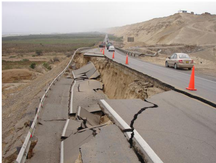
Figure 1.7. Deep sliding of road embankment in 2007 Pisco Earthquake, Peru (Photo credit: Ing. Jack Lopez)
