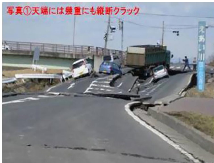
Figure 1.4. Left embankment at Fuchishiri-jyoryu of the Eai River (27.6 km). (Courtesy of Kitakamigawa-Karyu River Office Tohoku Regional Bureau of MLIT, 2011).
