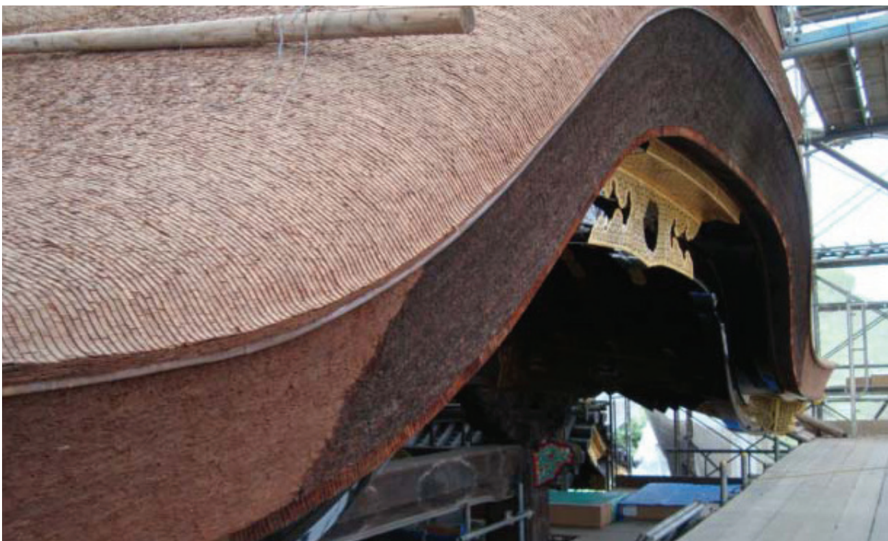
Kyoto. The restoration site of the Imperial gateway in Nijo Castle. June 25, 2013. Detail of the kara-hafu. The dark area is not restored. (2013 © Olimpia Niglio).
