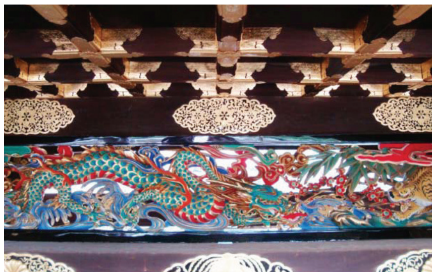
Kyoto. The restoration site of the Imperial gateway in Nijo Castle. July 30, 2013. The copper decorations and the wooden sculptures (three-dimensional) after the restoration (2013 © Olimpia Niglio).
