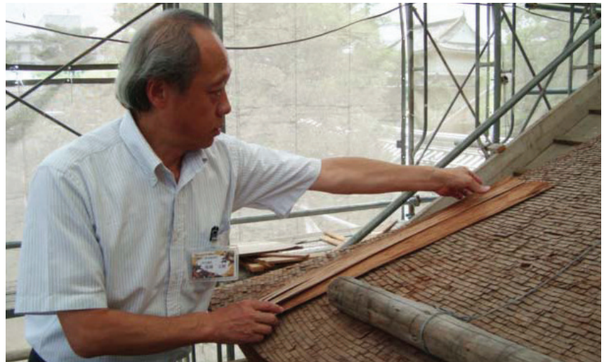
Kyoto. The restoration site of the Imperial gateway in Nijo Castle. June 25, 2013. The Architect Goto describes the restoration of roof with bark of the cypress. (2013 © Olimpia Niglio).
