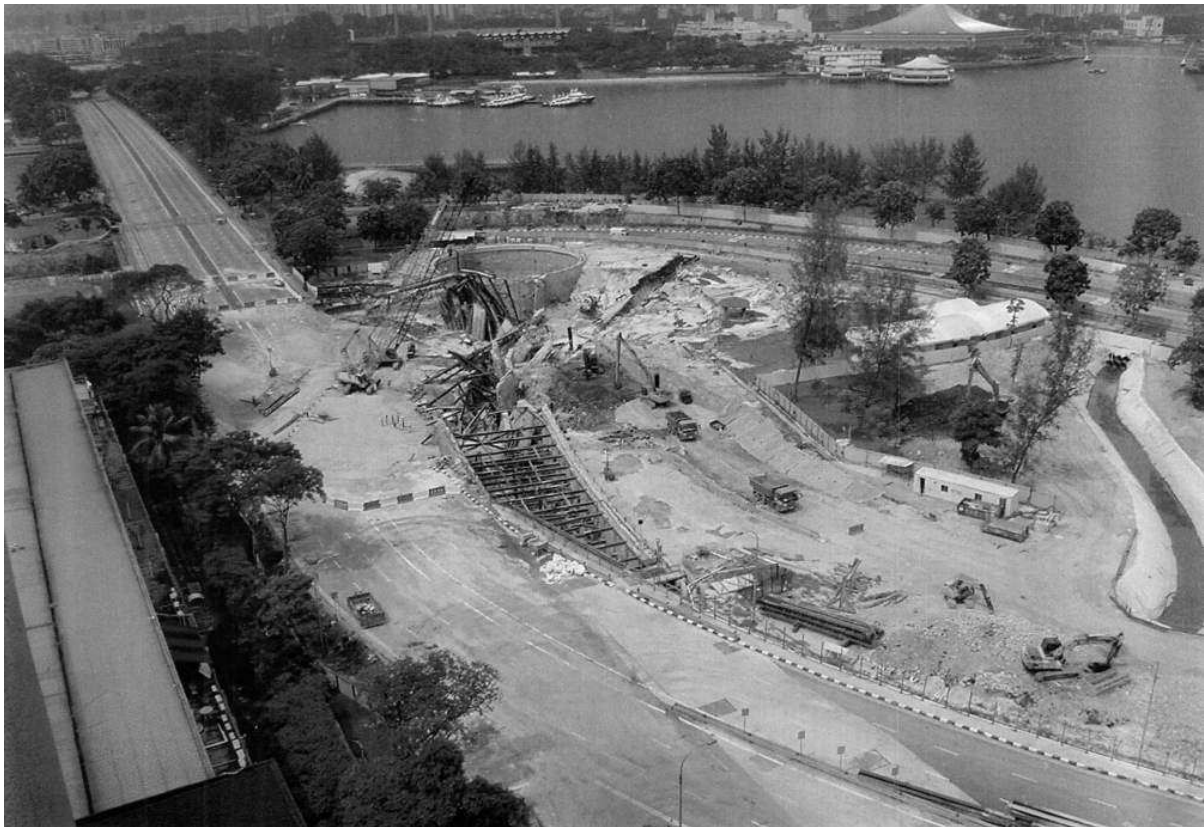
Fig. 3 Oblique view of the site to the east after the collapse.
