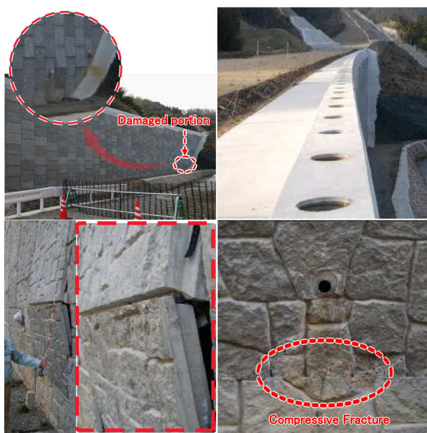
Fig. 4 Severely damaged portion.
