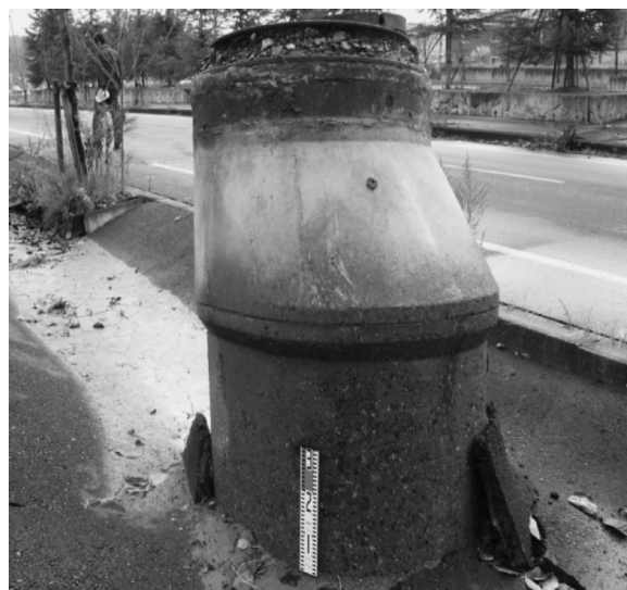
Fig. 1. Uplifted manhole after the 2004 Niigata-ken Chuetsu, Japan, earthquake
