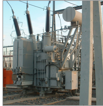
Fig 2.12 Power electric transformer
