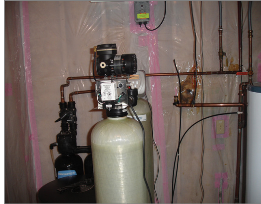
Fig 2.21 Damaged chlorination unit
