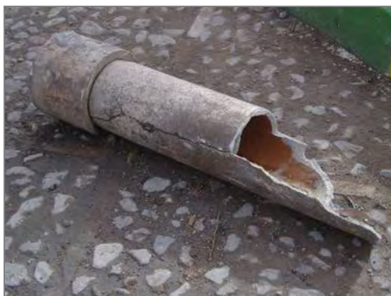
Fig 2.18 Damaged asbestos cement water pipe (IEEE)
