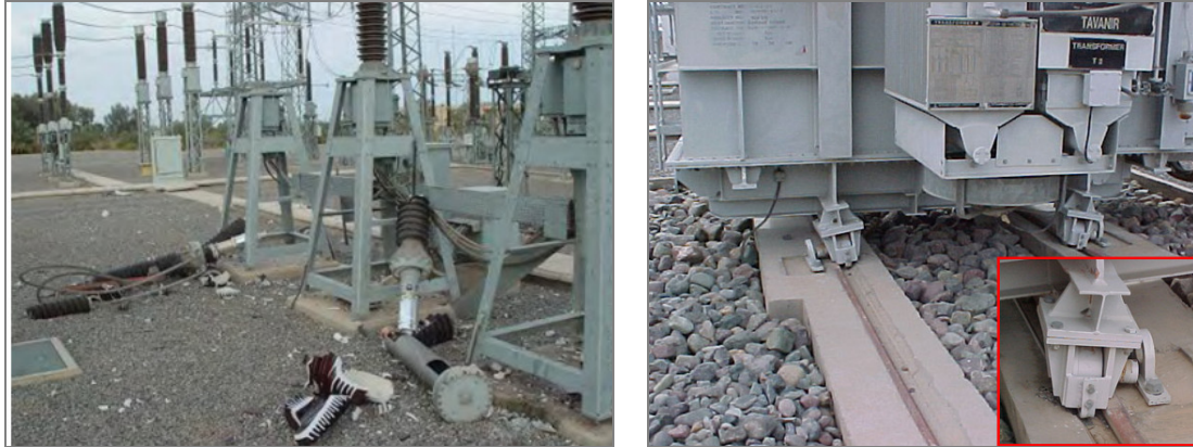
Fig 2.23 Damaged porcelain insulators and bushings, damaged foundation of 230 kV transformer
