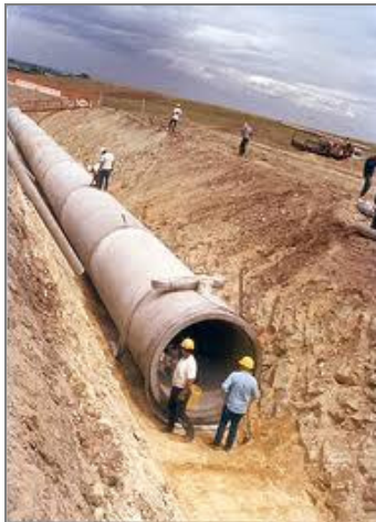
Fig 2.6 Water transmission main
