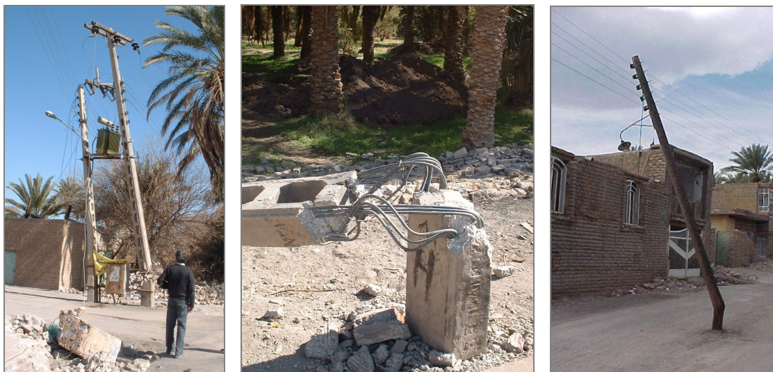
Fig 2.22 Damaged electric transmission concrete poles, distribution concrete and wooden poles
