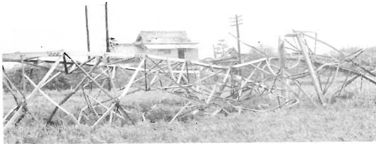
Fig. 1. Collapsed steel tower due to typhoon.
