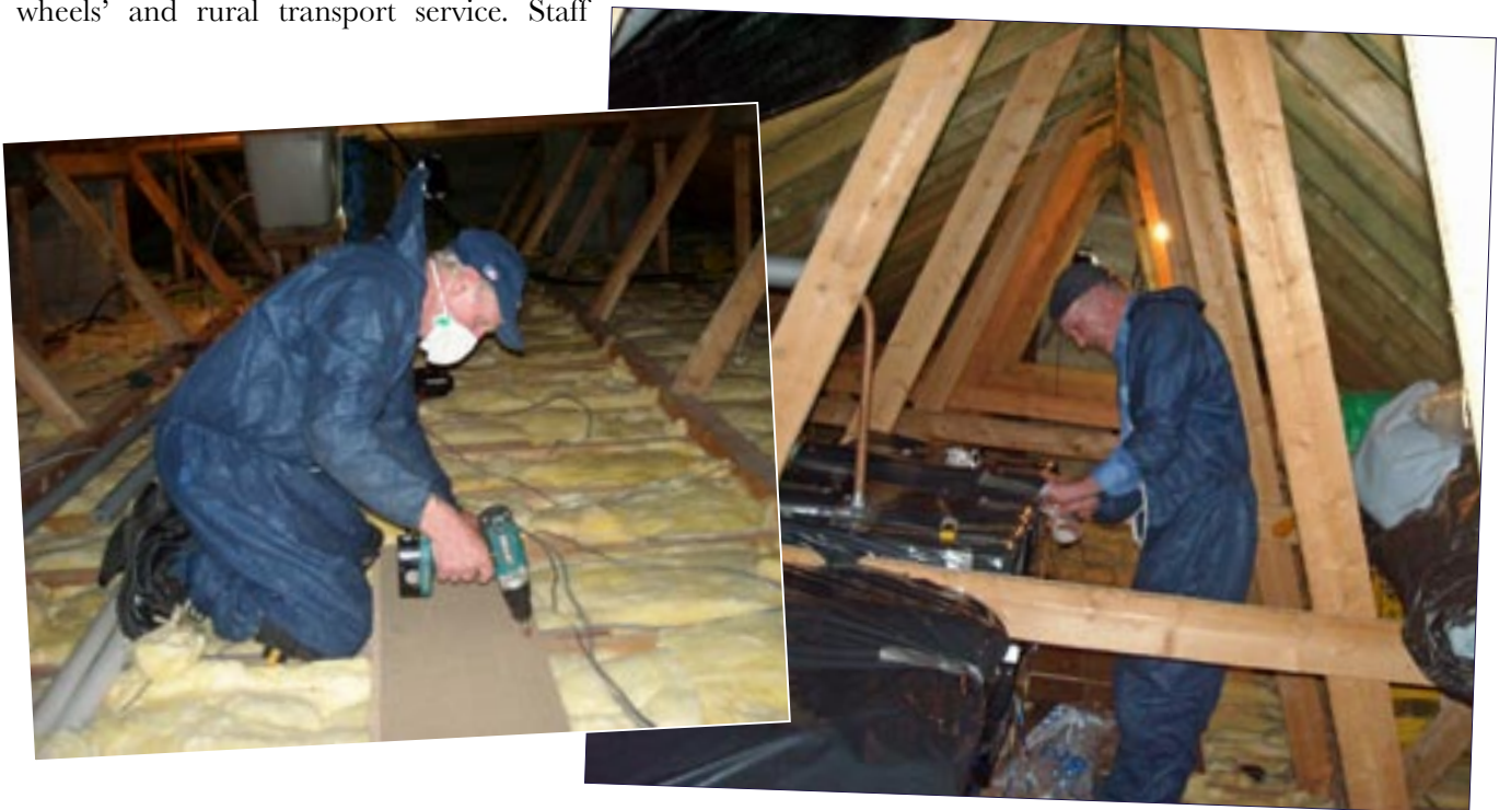
• Fig. 9 CSP participant Michael Enright fitting walk boards in an attic as part of the Warmer Homes Initiative. RSS participant Tim Enright insulating a cold water tank (Photos: IRD Duhallow).
