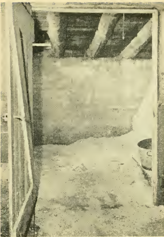
Fig. 42. A view from the stable alleyway looking into one of the sawdust storage bins.
