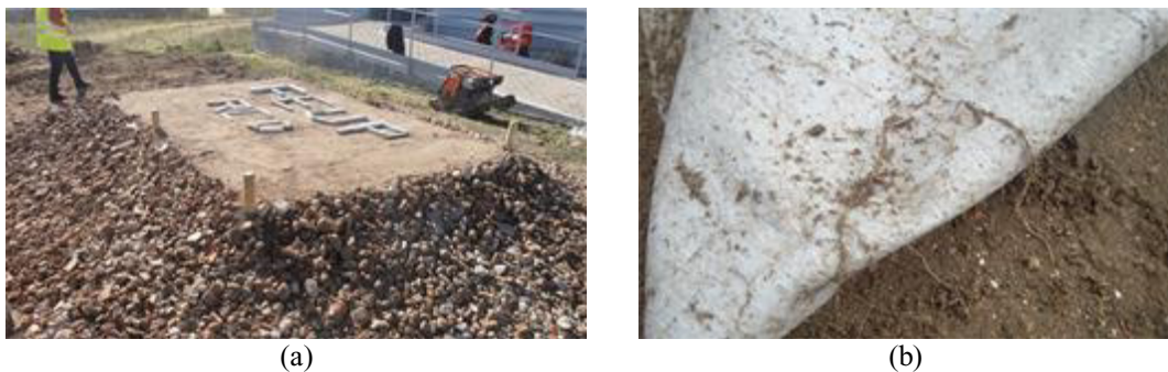
Figure 2: Trial embankments: a) one of the embankments at the end of construction; b) plant roots crossing the geotextile during exhumation.
