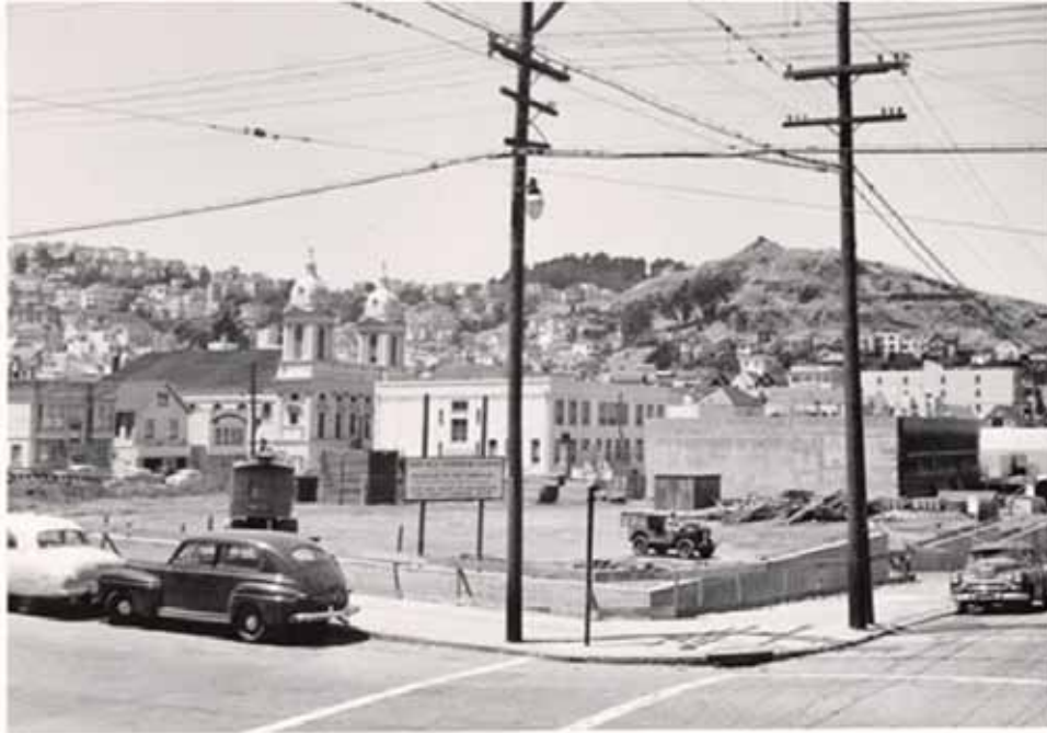
Figure 106. The Eureka Valley playground and recreation center under construction, ca. 1954. (AAE-0012, San Francisco History Center, San Francisco Public Library)
