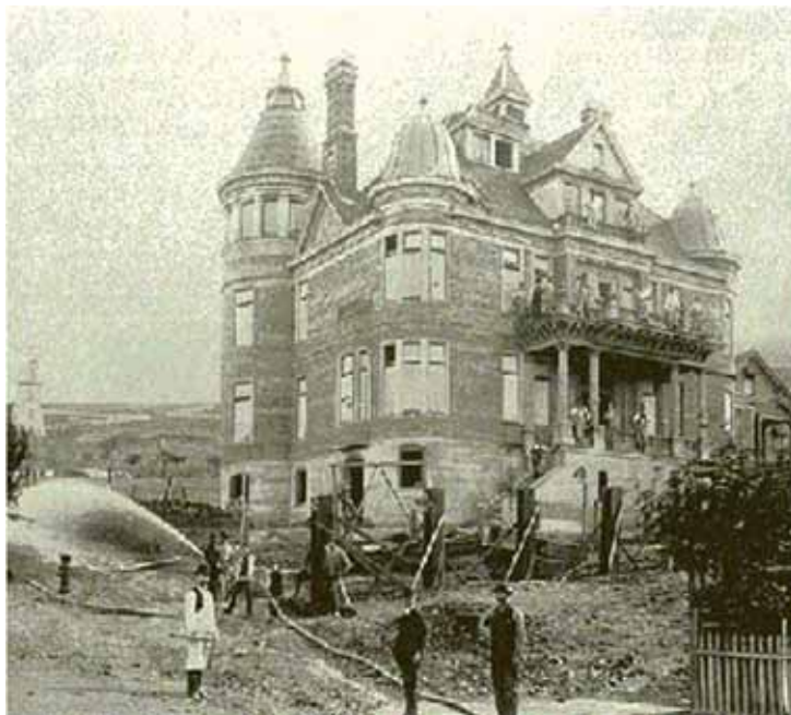
Figure 59. Alfred Clarke's home on Douglass Street under construction with demonstration of his water system pressure in foreground. (Private Collection, San Francisco, CA; published online at http://FoundSF.org/index.php?title=Alfred_%22Nobby%22_Clarke:_The_Police_Department%27s_%27Emperor_Norton%27 )
