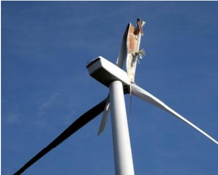
Figure 2-14 Complete structural failure of rotor blade due to excessive winds (Dongsheng, et al., 2015)
