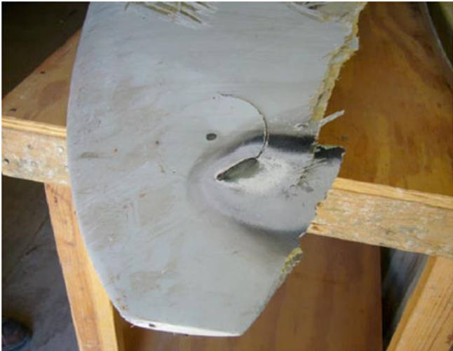
Figure 2-15 Damage on rotor blade tip due to lightning strike (Dongsheng, et al., 2015)
