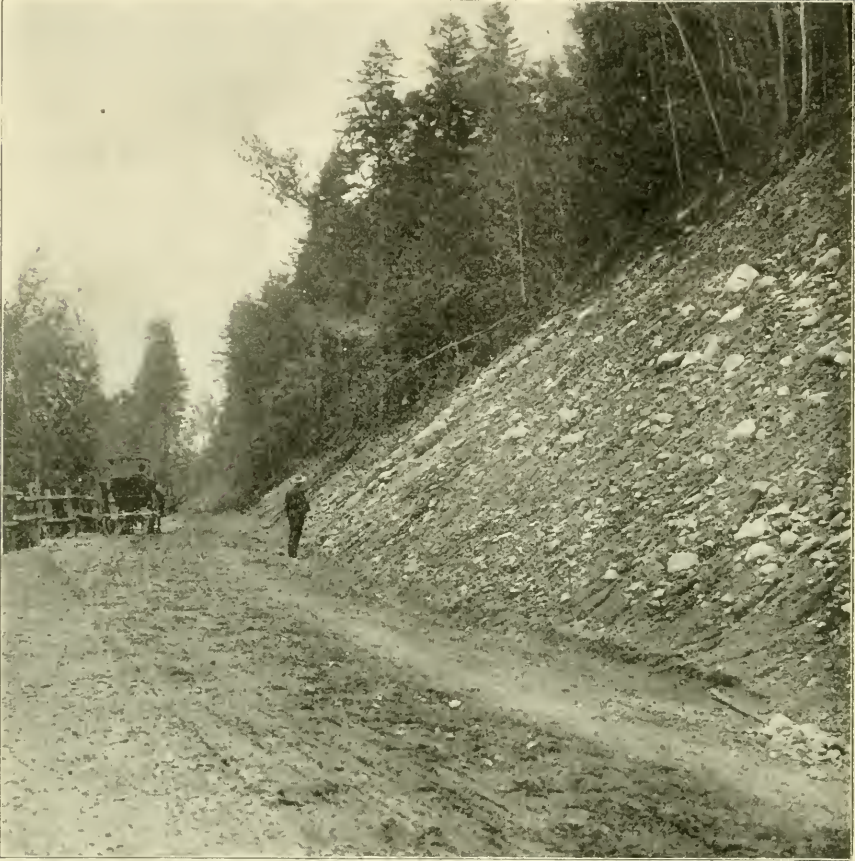
Section of Road between Fabyans and Twin Mountain House, Showing Side-Hill Cut.
