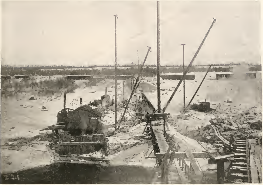
Winter view, looking across the river. Construction was scarcely interrupted all winter.
