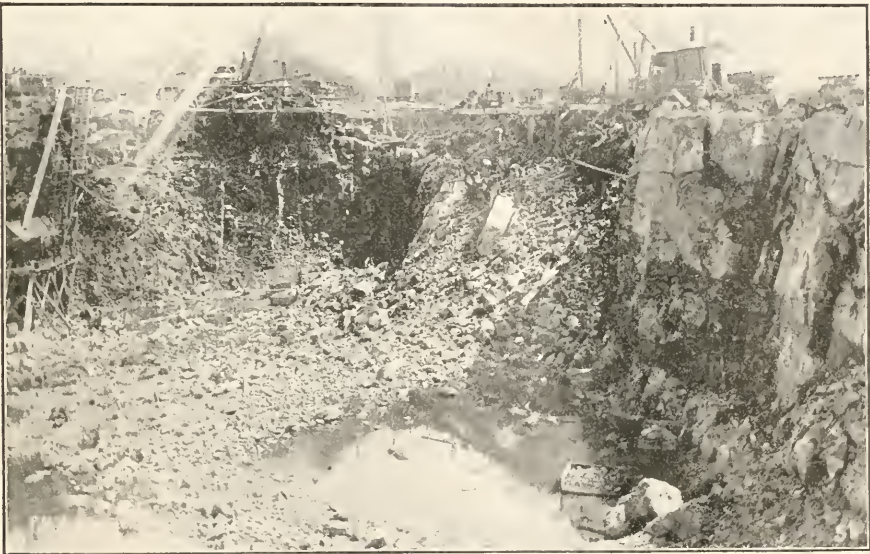
Henderson's point, showing the rock excavation, about sixty feet in depth and carried to near the water line on three sides, September 1, 1903.
