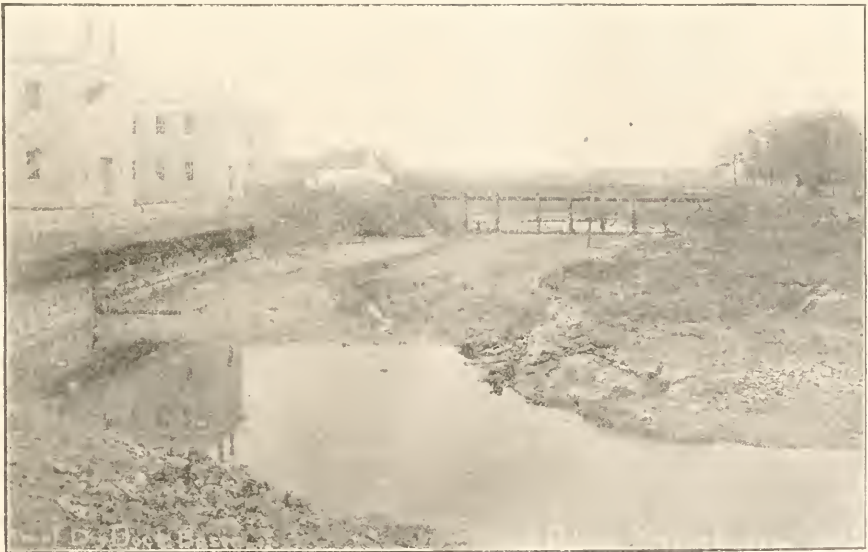
Site of the new dry dock, showing the bridge connecting Savage's island, taken May 19, 1900.
