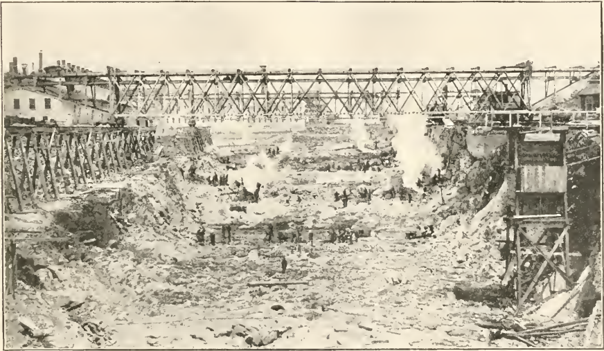
Site of dock partly excavated, showing the numerous steam drills used for blasting, May 2, 1901.
