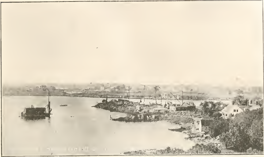
Henderson's point at the commencement of the excavation, showing the channel since then filled in, October 7, 1902.
