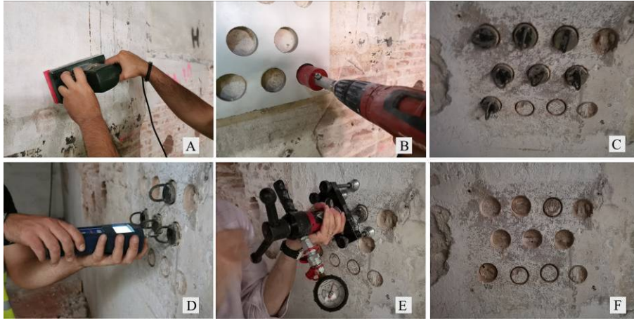
Figure 3: Pull-off test operation: (A) removing the surface paint layer with a mechanical sanding, (B) drilling the plaster until reaching the masonry substrate using a 50 mm diameter core bit, (C) sticking the metal discs, (D) manual dynamometer, (E) mechanical dynamometer support, and (F) failure of plaster substrate.
