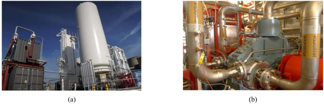
Figure 11. (a) External; and (b) internal views of the 350 kW e /2.5 MWh LAES pilot plant [75].
