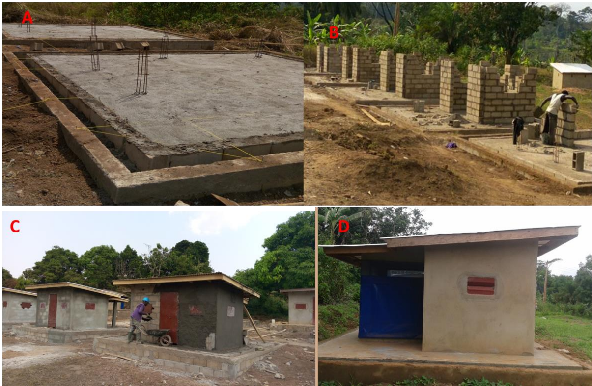
Figure 4.3: Different steps of hut construction. A) Huts are built on a concrete base surrounded by a narrow moat to exclude scavenging ants. B) Construction following the plan and the dimensions. C) Plastering of walls made from a mixture of cement. D) The final version of the hut.
