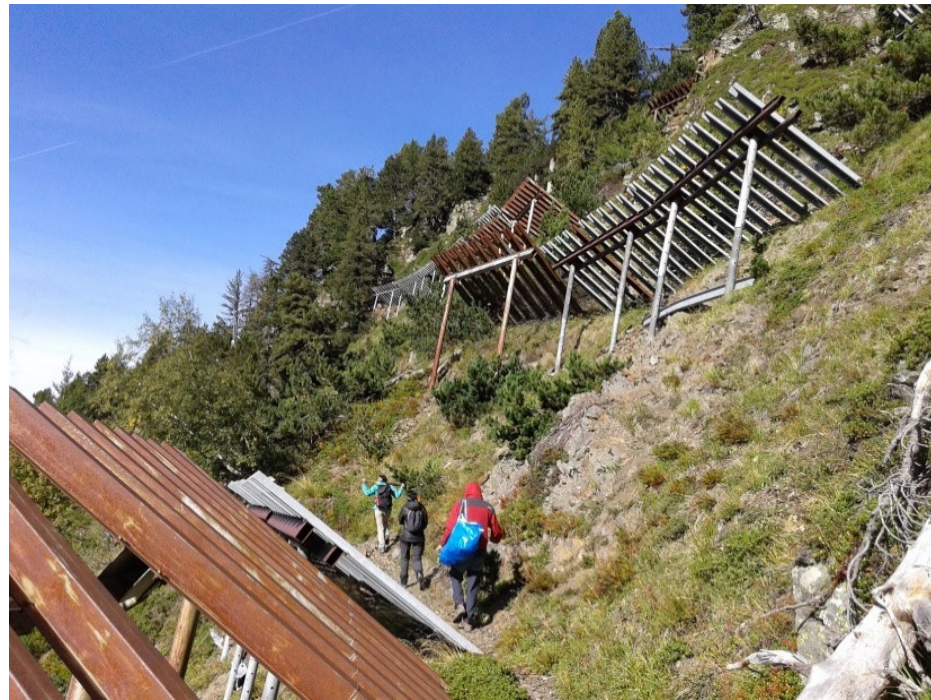
Figure 1. Anti-avalanche structures in Thiel corridor above Barèges.
