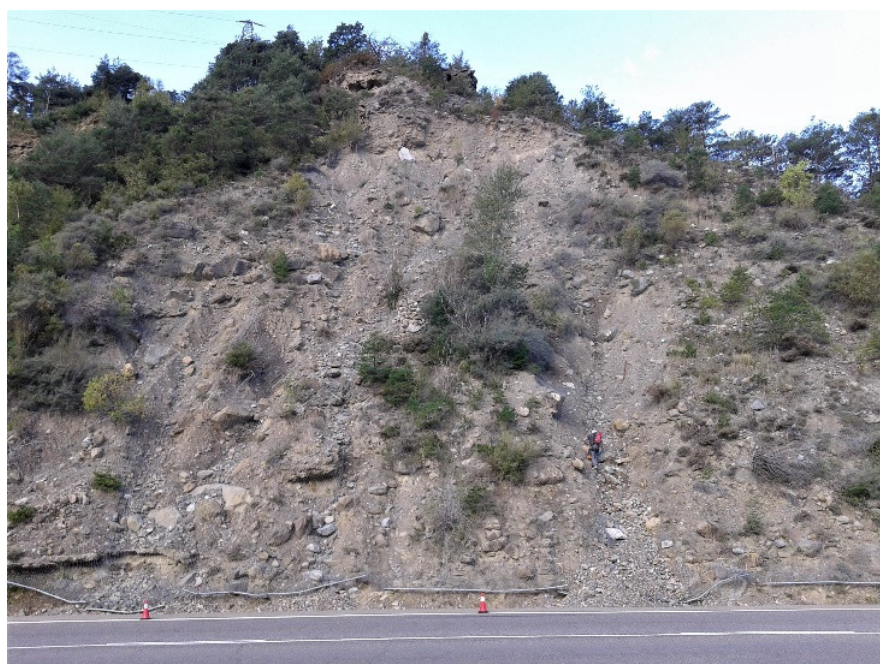
Figure 3. Sediment instability in the Santa Elena road cut.
