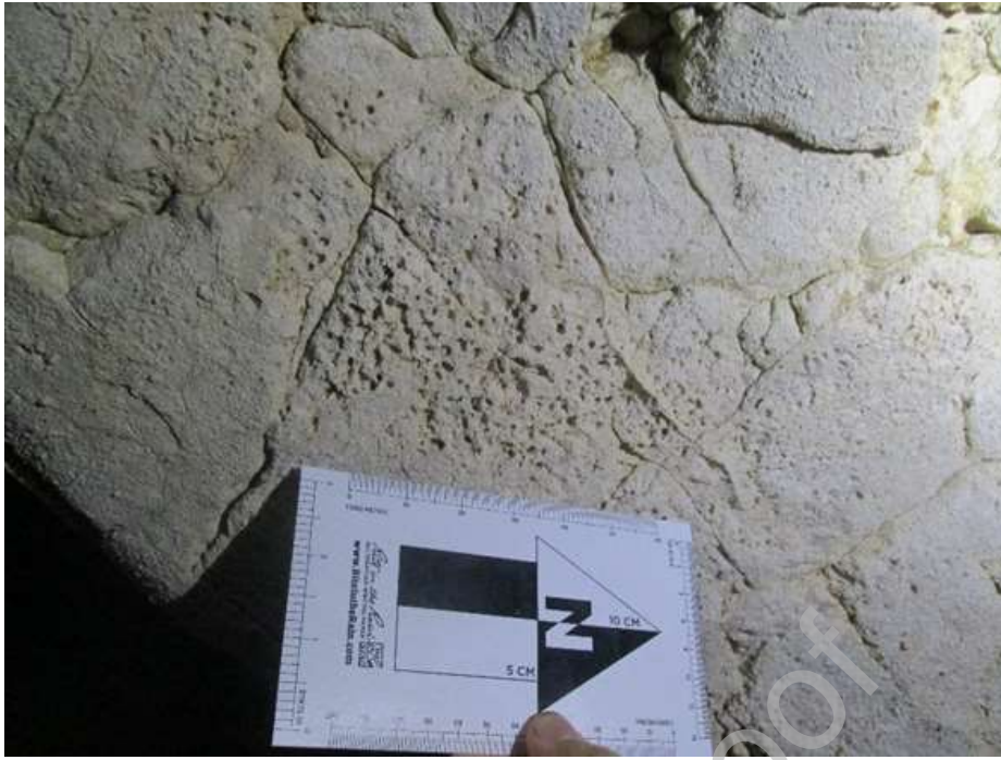
Figure 1: Condensation corrosion dissolution features on the limestone ceiling in Tomo Passage, Waitomo Glowworm Cave. Photo from Ingrid Lindeman.
