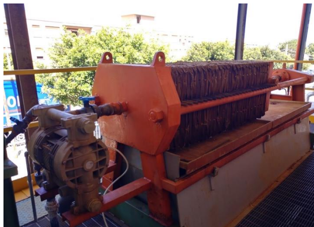
Figure 5-10 Press filter for the iron hydroxide separation.
