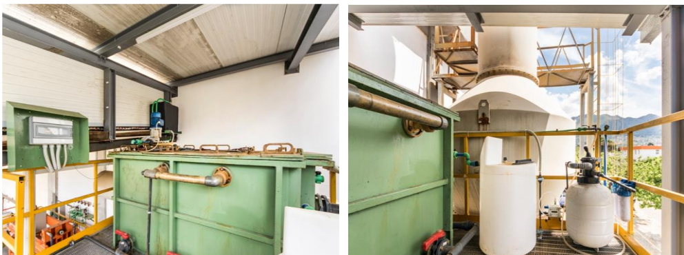
Figure 5-4 Pre-treatment section: (on the left) heated oil separator and (on the right) activated carbon filter.
