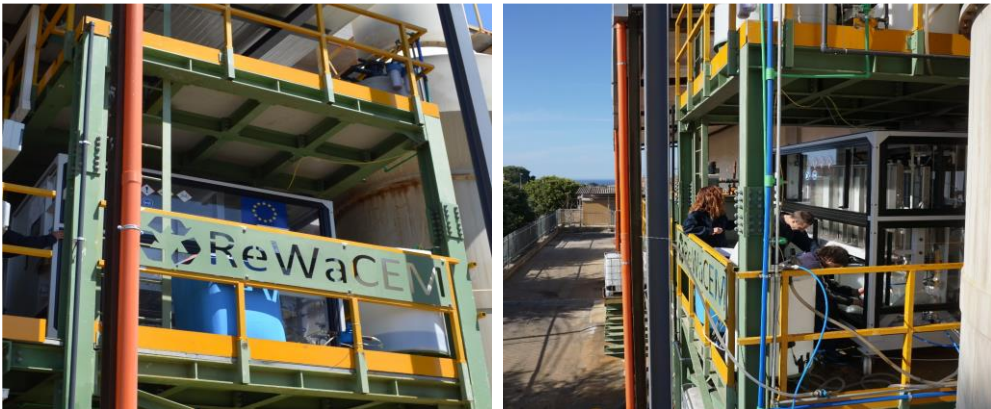
Figure 5-3 Demonstrator unit installed on the first floor at Tecnozinco hot-dip galvanizing plant (Carini (PA), Italy).
