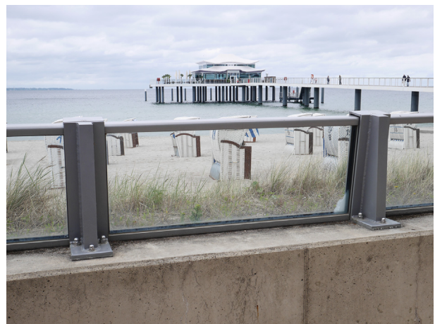
Fig. 3. The scenically integrated protective wall in Timmendorfer Strand (Photographed by Nico Stelljes in June 2015).
