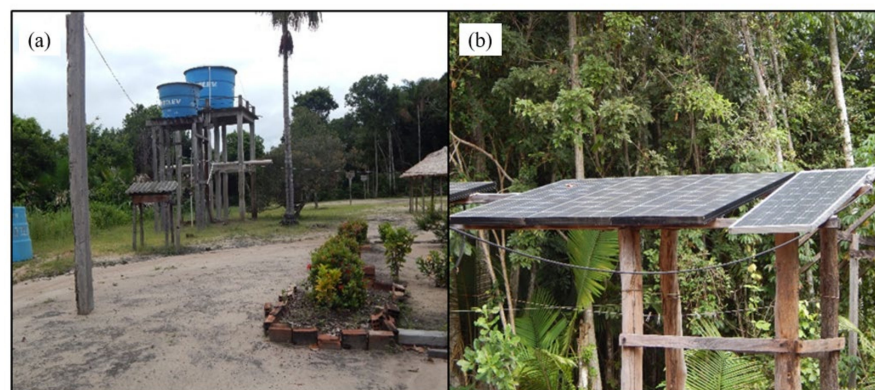
Figure 8. Infrastructure in two communities at RESEX Tapajós-Arapiuns, Pará, Brazilian Amazonia: (a) microsystem in the community of São Miguel; (b) solar panel in the community of Maripá.
