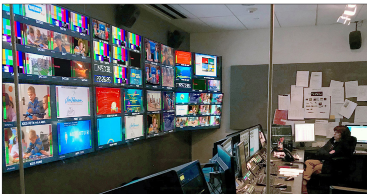
The Master Control room at WGBH (now GBH) in March 2020. The monitors on the wall display the outgoing broadcast signals for 13 channels in and around Boston.
