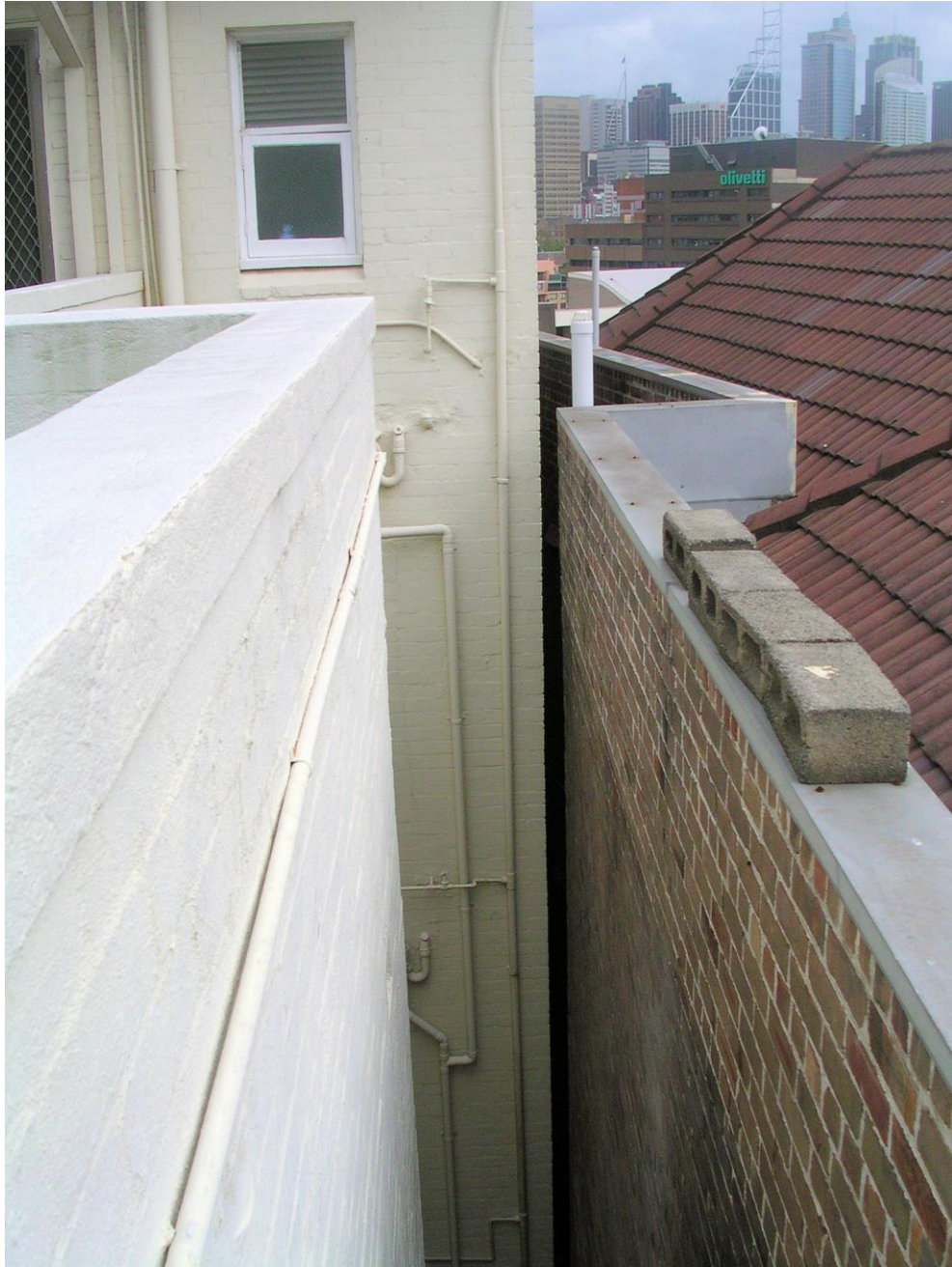
Figure 7: Roof gap, haunting drops (author's photo)
