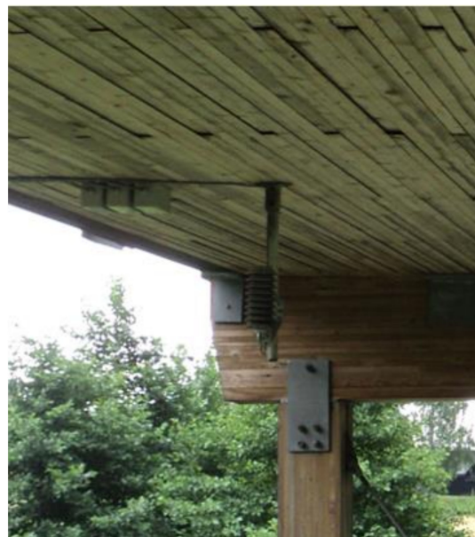
Figure 5. Sørliveien Bridge. Detail of the bottom deck with the monitoring equipment.
