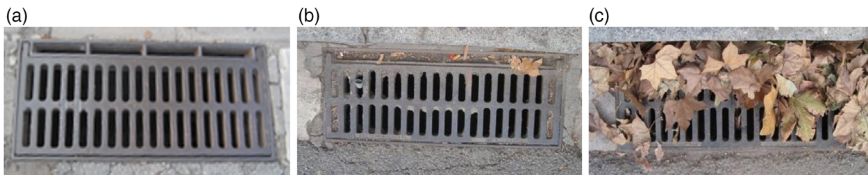
FIGURE 1 (a) Clean and (b and c) clogged inlets
