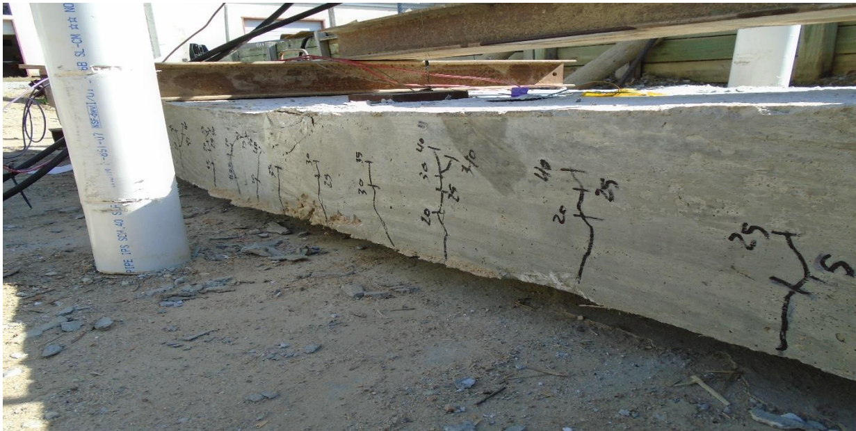
Figure 2-11. Cracks patterns of deck No. 5-2 at failure.
