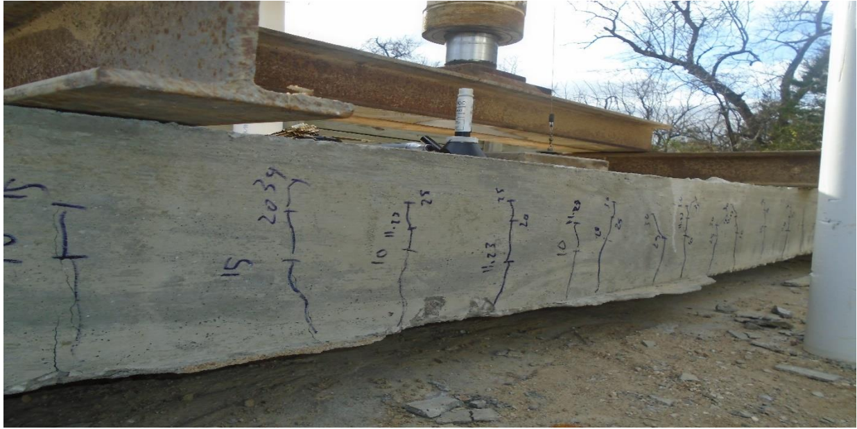
Figure 2-10. Cracks patterns of deck No. 5-1 at failure.
