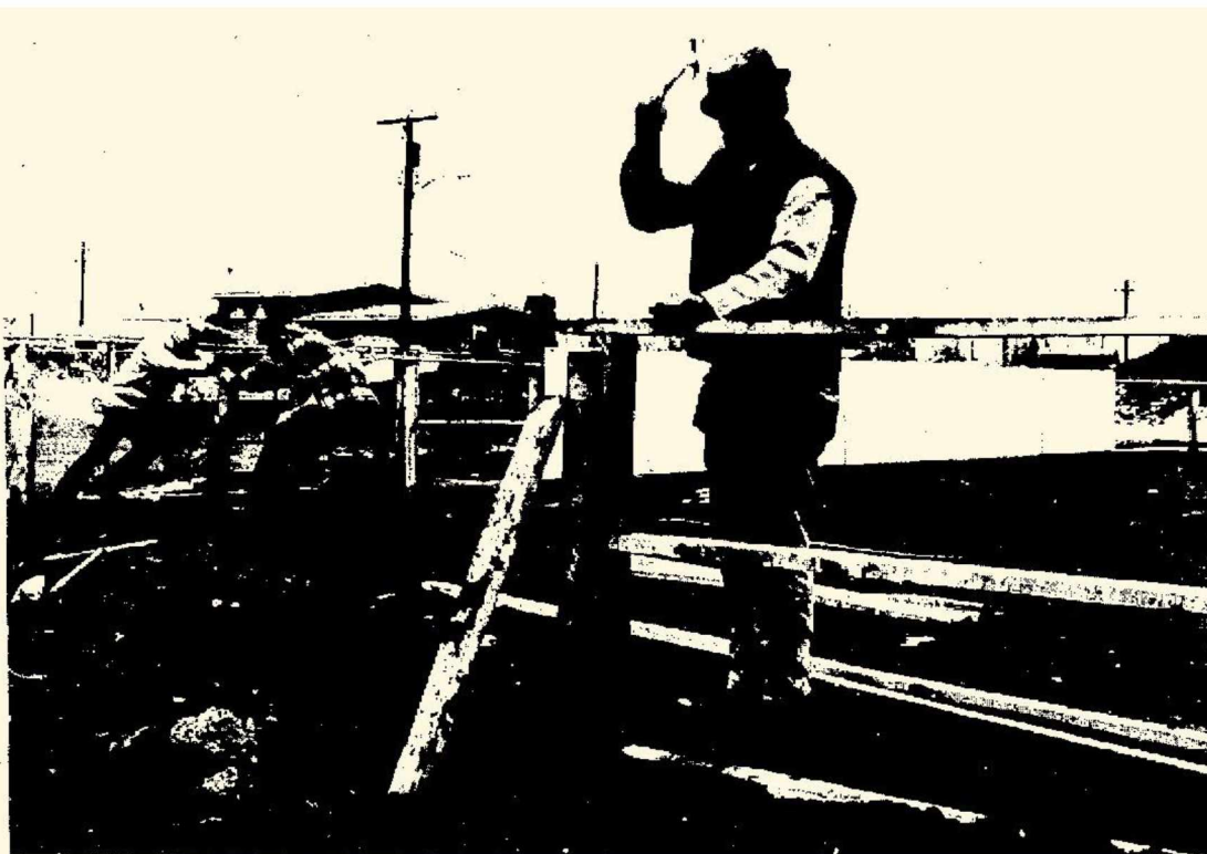
READY FOR HOCKEY SEASON —Richard Barnett works on framing for Barnette Elementary School hockey
