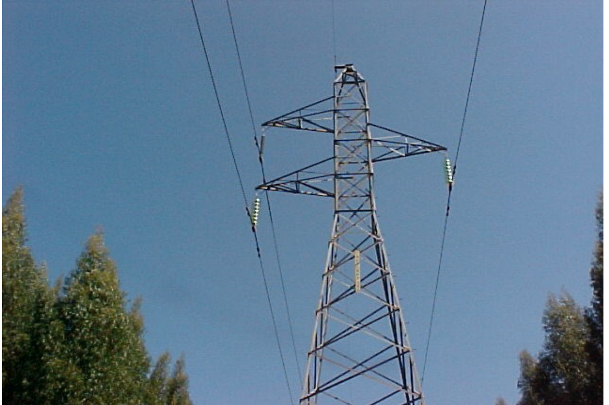
Figure 5.3 Typical tower for HVAC transmission lines.
