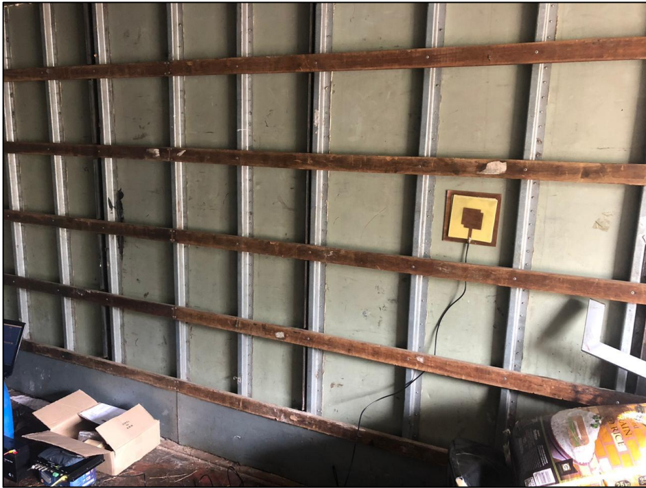
Figure 41: Placing of the UHF RFID antenna connected to a 50-ohm cable.
