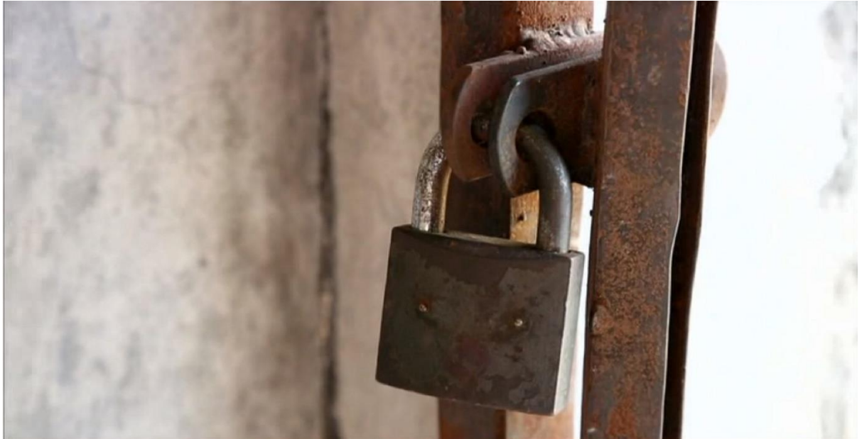
Main gate of this factory was locked during a fire incident. Image source: Dying for a Bargain (2013), copyright permission obtained from the producer.
