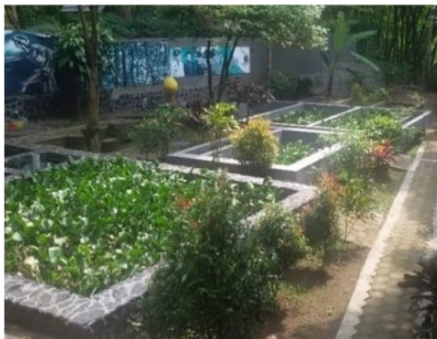
Figure 1. The condition in IPAL Komunal Tlogomas
