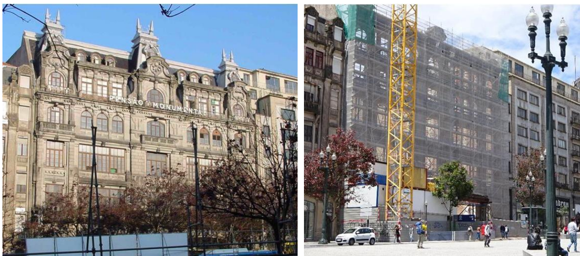
Figure 8 – Monumental Guesthouse before the works (Esmeralda Paup rio, 2004) and during intervention (Teresa Ferreira, 2016).
