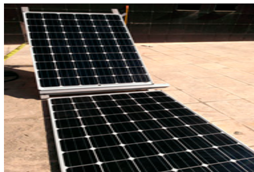
Figure 1. Installed panels for the experiment at study.
