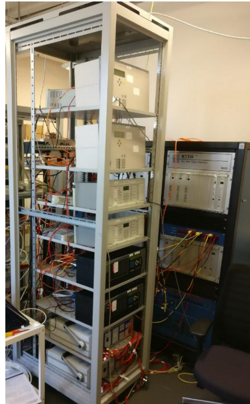
Figure 2: Selection of protection relays, RTDS simulator, and injection equipment
