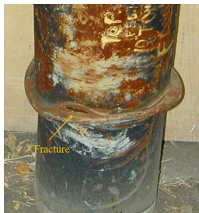
Figure 1.3: Fractured Field Pipeline of WestCoast Energy Inc. (Courtesy of WestCoast Energy Inc.)
