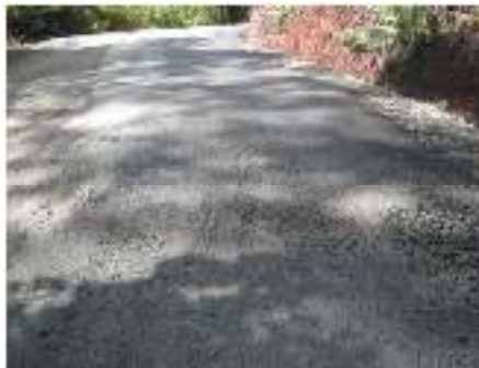
Gambar 2.5. Retak halus ( hair cracking )
