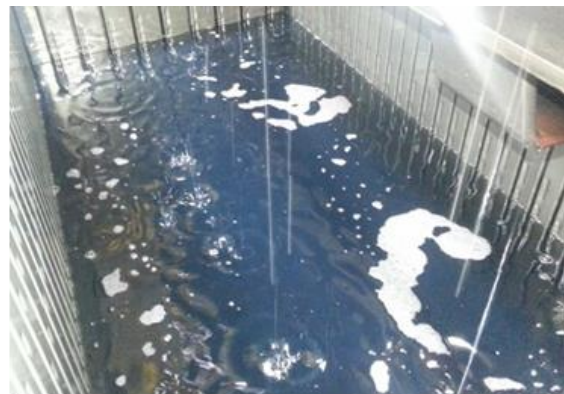
Fig. 13: Transformer oil degradation. Fresh oil (according to the manufacturer's characteristics) is pale yellow and transparent.
