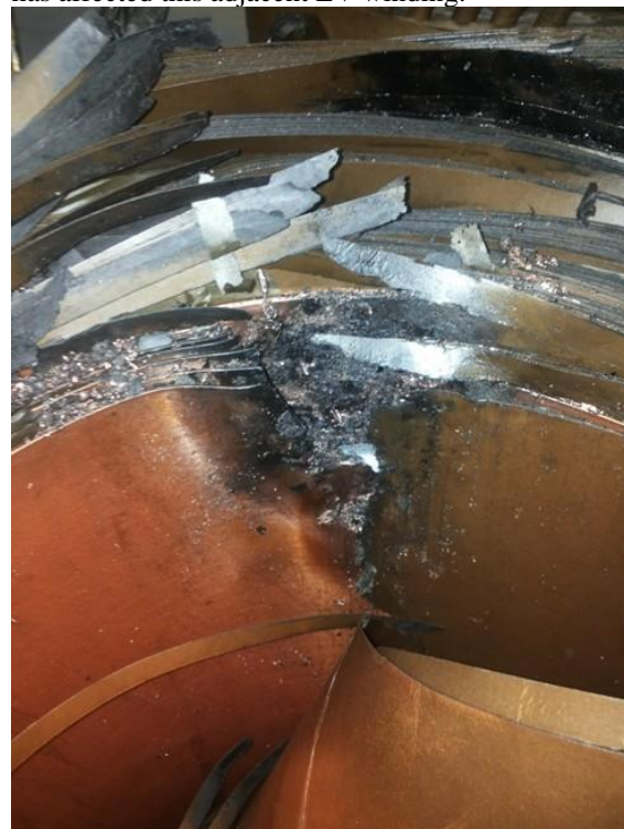
Fig. 10: Detail of the location of the interturn short circuit on the LV coil of the transformer. The interturn short went through 9 layers of the winding.
