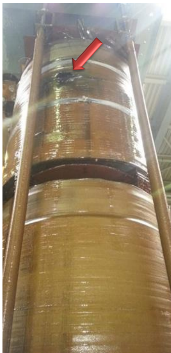
Fig. 5: Damaged HV coil visible after removing the transformer from the oil sump. The fault on the HV winding is located approximately in the middle of the column.
