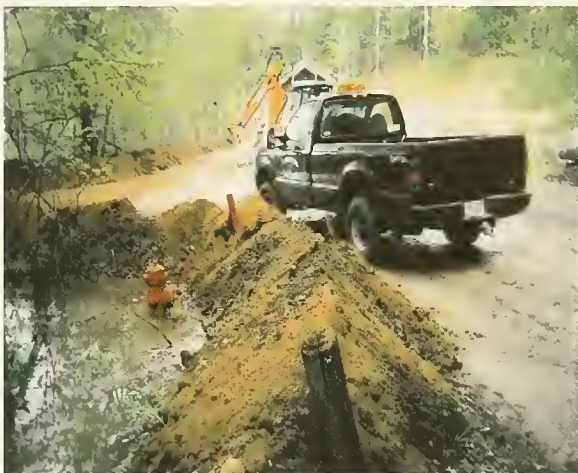
Village Water So. Well Pump Station
