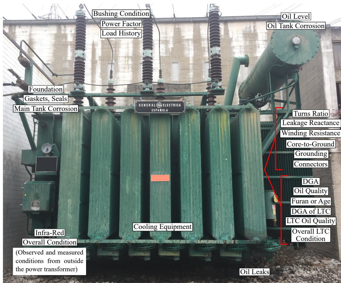
Figure 1. Locations of condition parameters used to calculate the HI of the transformer.
