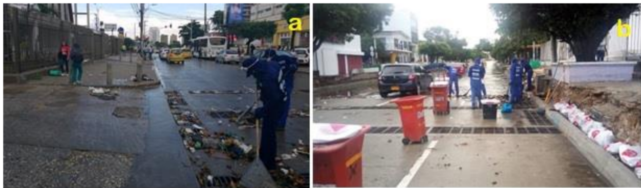
Figure 7. (a,b) Government actions to avoid obstruction of recently constructed stormwater runoff channel. (Source: Mayor of Barranquilla, 2020).
