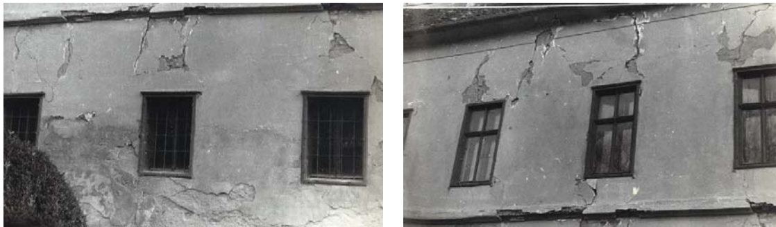
Figure 12: Vertical and diagonal shear cracks detected in the South façade of the case study building [16].
