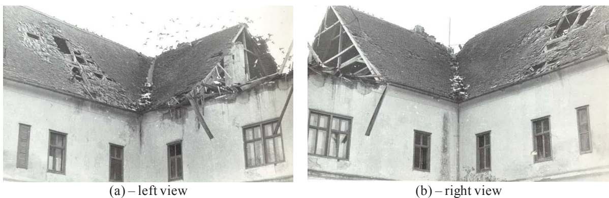
Figure 13: Failure mechanisms observed in the internal court of the case study building [16].
