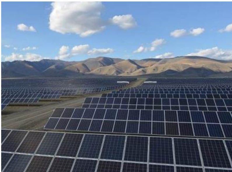
Pic 2.4 SPP based on photovoltaic modules and solar panels
