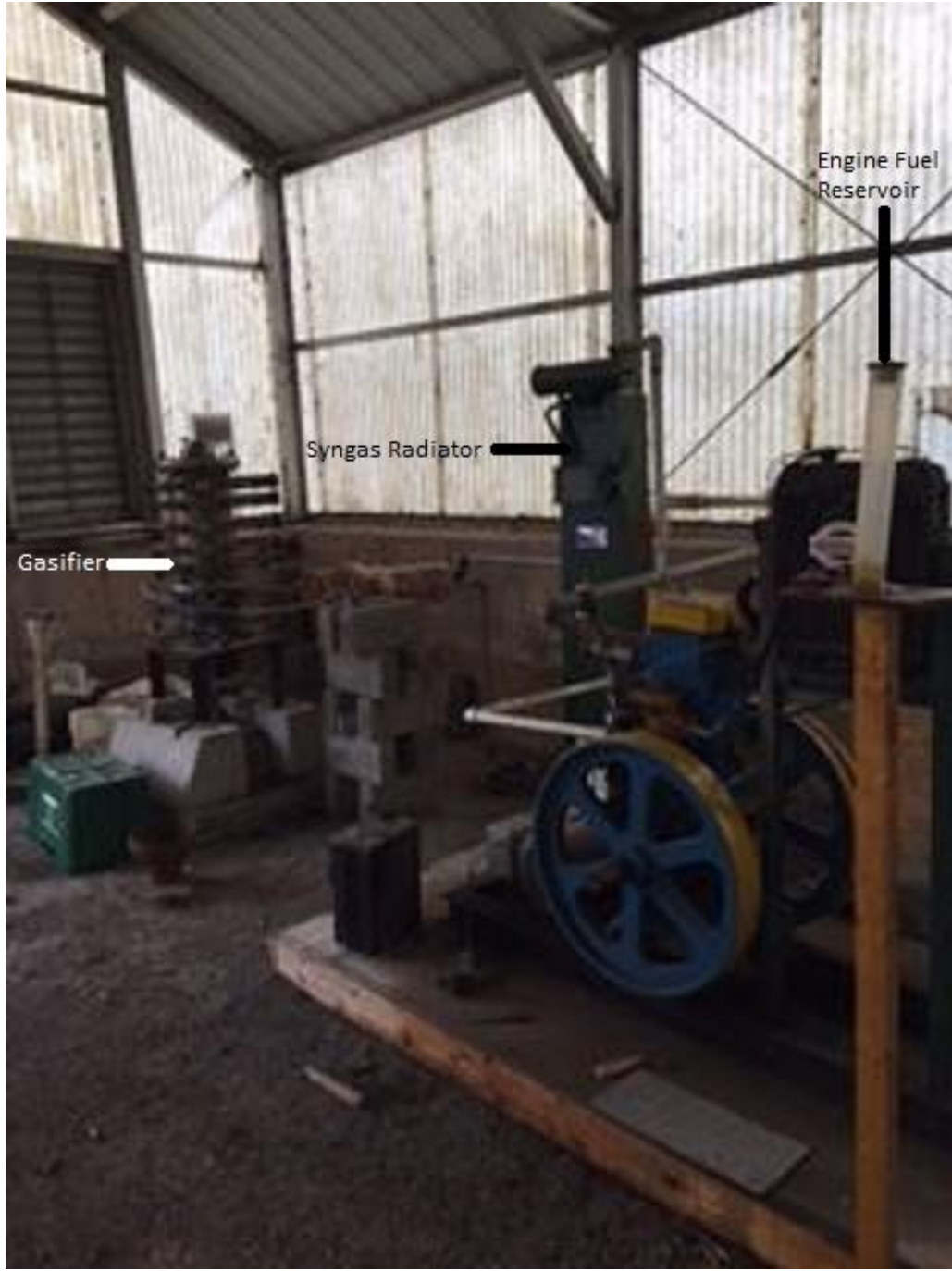
Figure 8. CERF Gasifier Genset System
