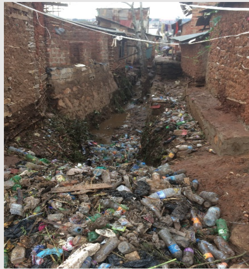
A major drainage channel in Namuwongo after heavy rain. (photo by Magdalena Bondos, LSHTM ©)
