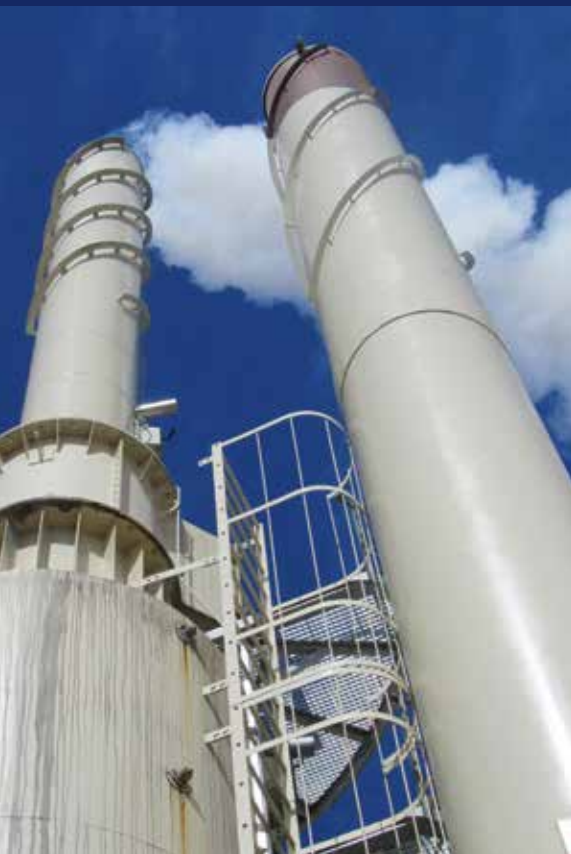
Biomass district heating plant in Ludza
