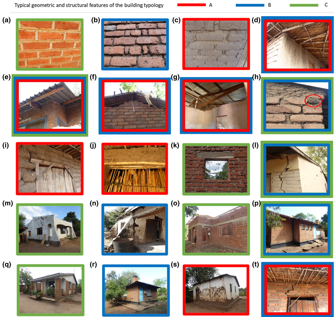
Fig. 6 Typical buildings in Malawi: a fired bricks with cement mortar; b fired bricks with mud mortar; c unfired bricks with mud mortar; d thatched roof; e light metallic sheets; f gable detached from the roof structure; g lack of connection between walls and roof system; h timber wall plates of circular section; i door frame showing absence of lintels; j bamboo lintel; k concrete lintel; l house with poor
